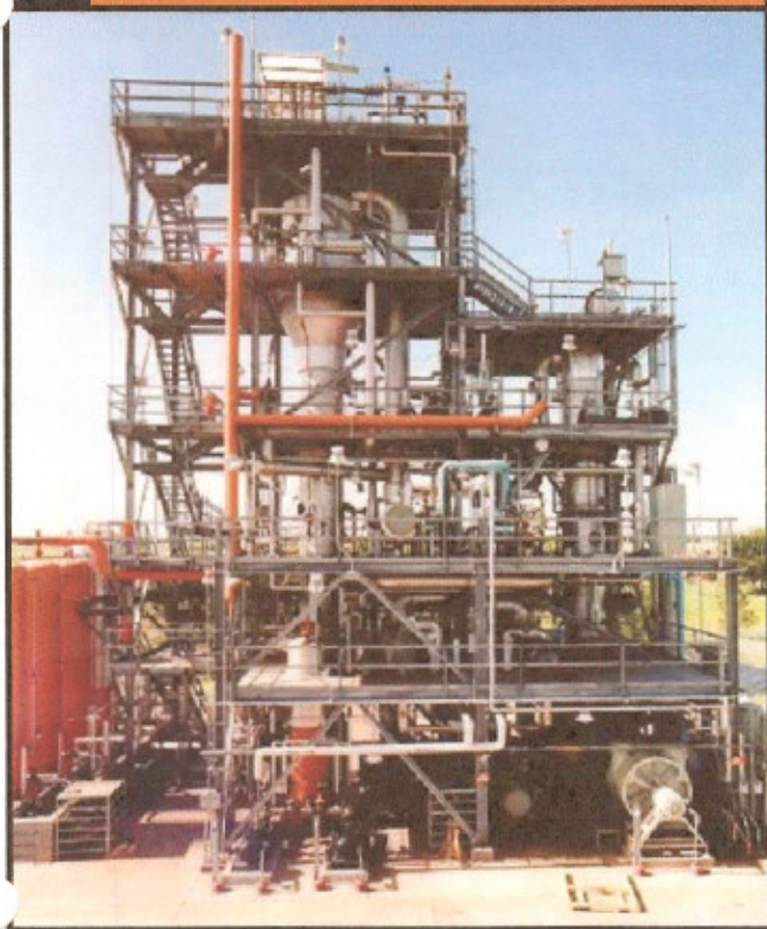
Figure 1. FRI has both high- and low-pressure commercial-size distillation columns.
